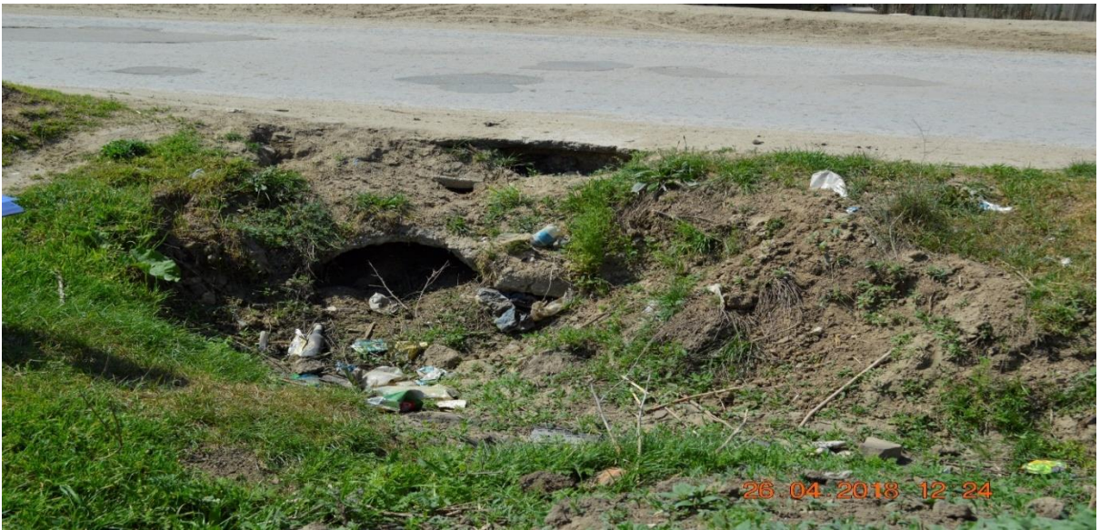
Figure 3.9.2. Silting an essential part of the culvert on km 13,400.
