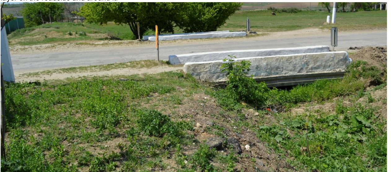
Figure 5.1.2.1. Silted culvert on km 6, 80
