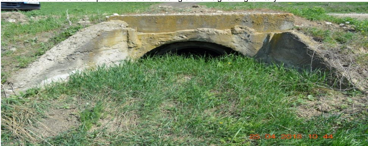
Figure 3.9.2. Silting an essential part of the culvert
