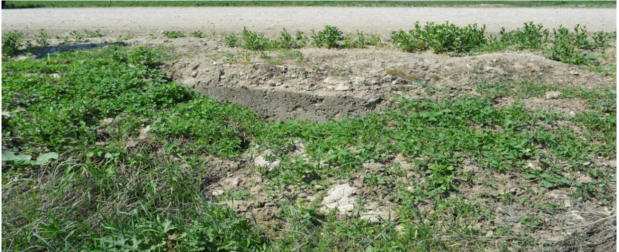
Figure 5.1.2. silted culvert on km 14,800
