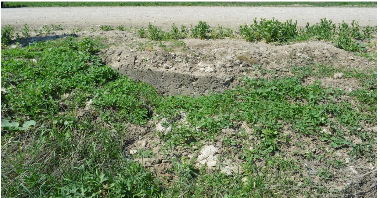
Figure 5.1.2.2. Silted culvert on km 14,800
