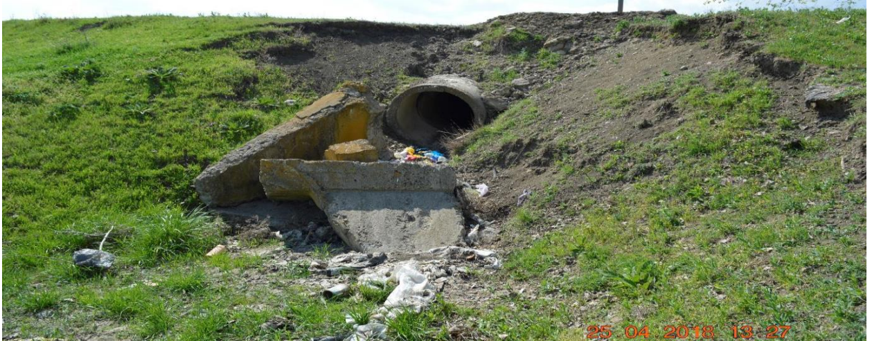
Figure 5.1.2.1. Downstream erosion of the culvert with partial degradation of the culvert
