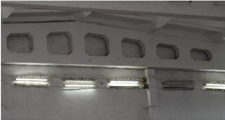
Photo 9 Lighting in the gym
