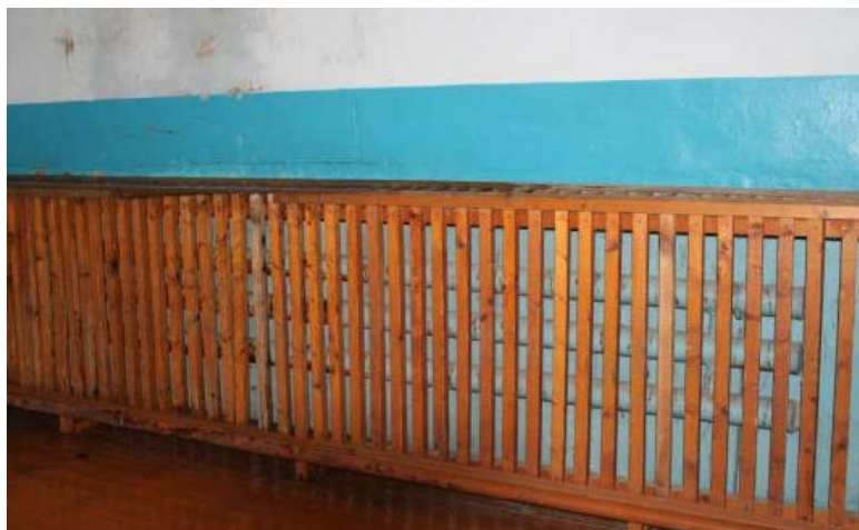
Photo 6 Tubular radiators in the gym
